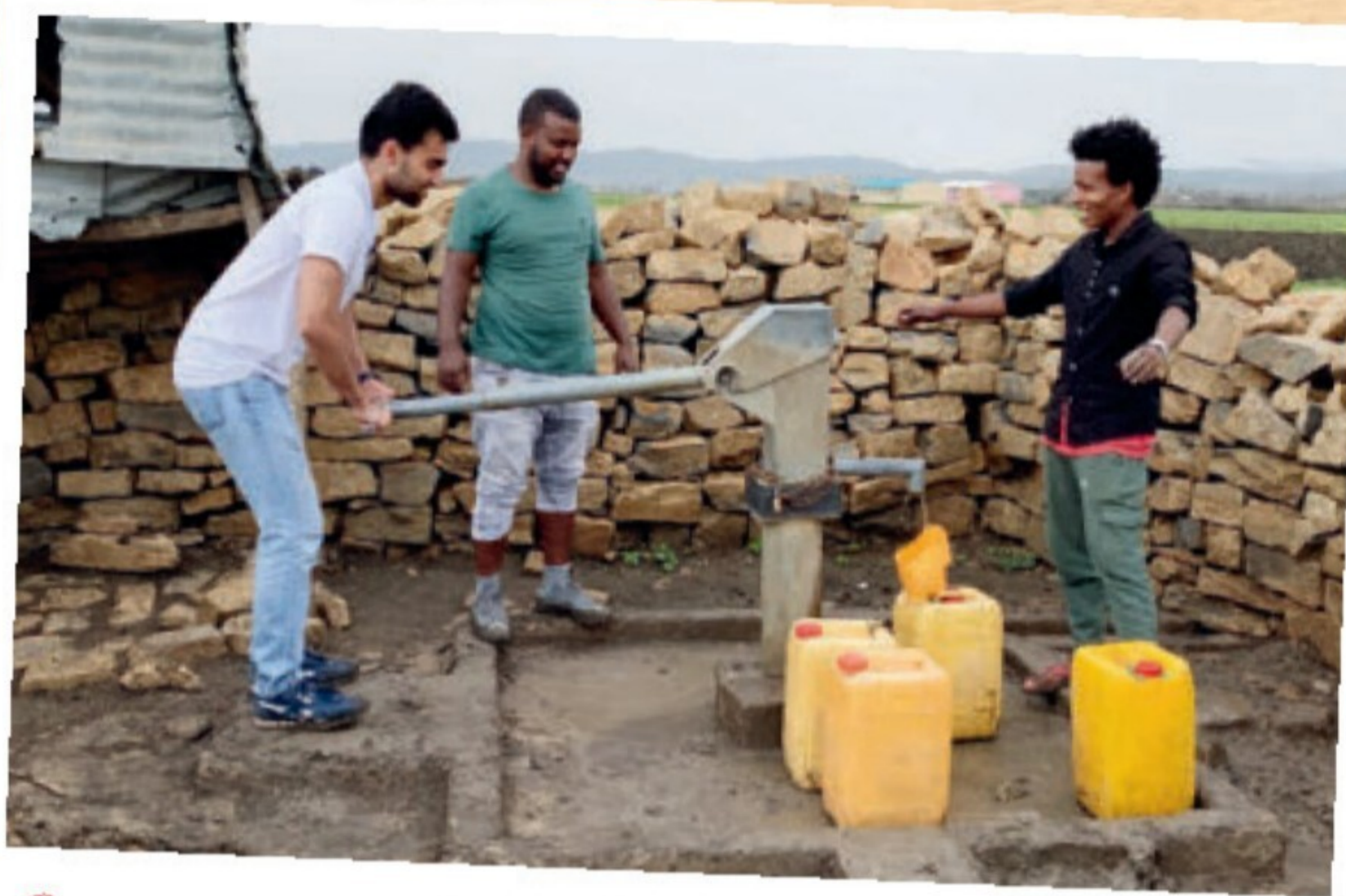
Prior to renovation, the building did not have running water, so team members had to walk 800 meters - about half a mile - to the village well to get water and then hire donkeys to carry it back to the construction site, where it was mixed with cement. At left: Team member Fahad Kazi pumping water at the well
