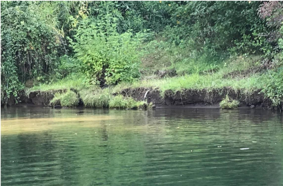
Figure 2 - Undercutting at Champoeg Park.
