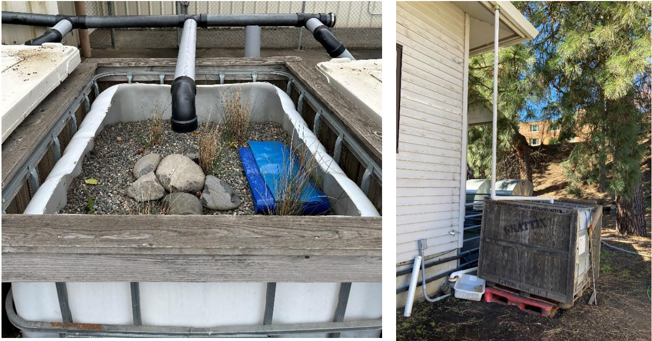
Figure 1. Photo of installed roof runoff filter (left: top view; right: side view).
