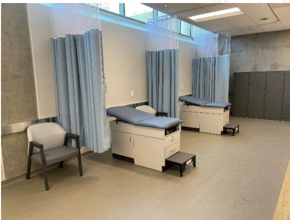
Nursing Simulation Center under construction looking at the Exam area of the Hospital Bed Unit.
