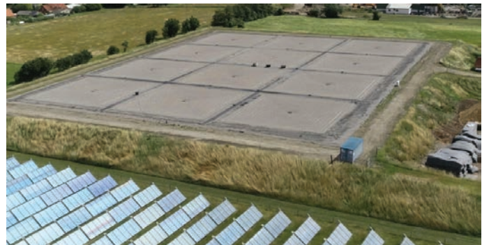
Figure 30: Flat Plate Solar Collector Plant.
